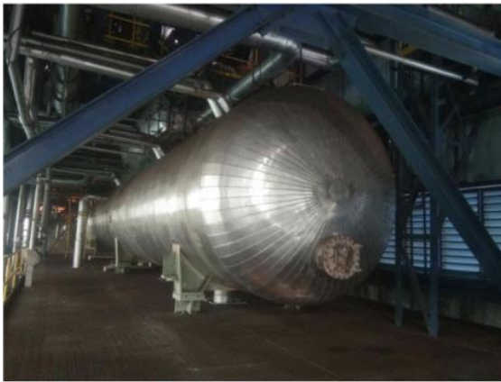
Gambar 3. 24 High Pressure Heater
