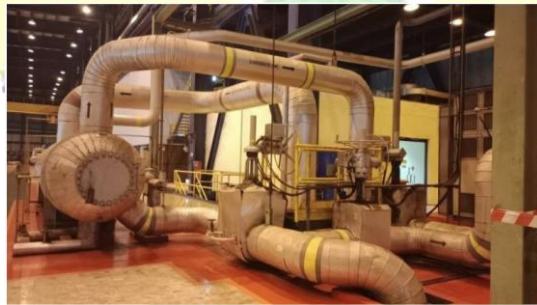
Gambar 3. 21 Low Pressure Heater
