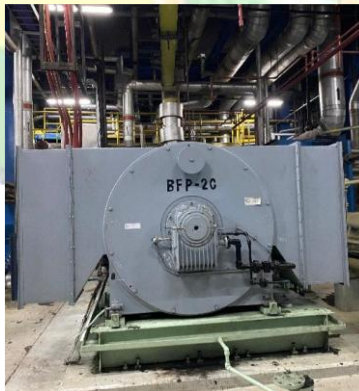
Gambar 3. 23 Boiler Feed Pump
