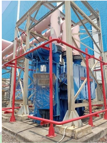
Gambar 4. 3 Transformator UAT 1B
