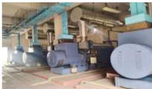
Gambar 2. 9 Generator set Terminal 2
