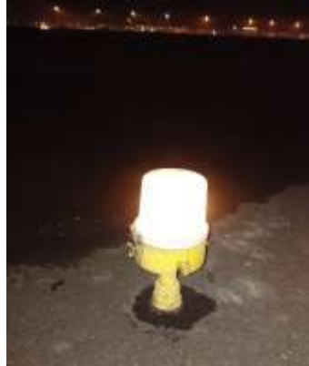
Gambar 3. 6 Runway Edge Light Elevated
