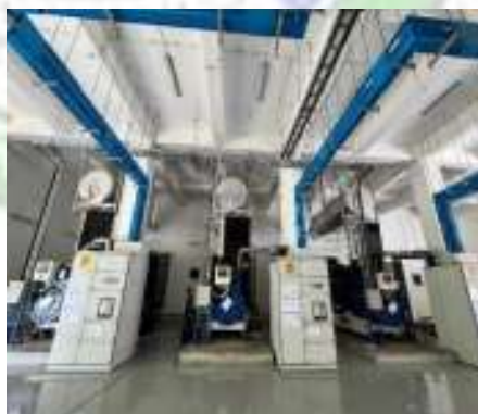
Gambar 2. 10 Genset Terminal RTT
