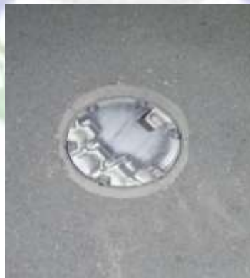
Gambar 3. 7 Runway Edge Light Inset
