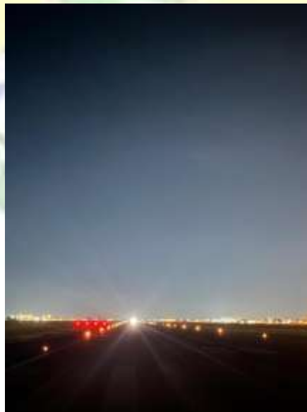
Gambar 3. 1 Airfield Lighting System (AFL)
