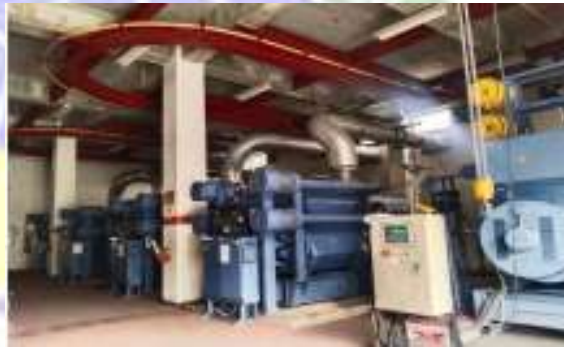
Gambar 2. 8 Generator Set Terminal 1
