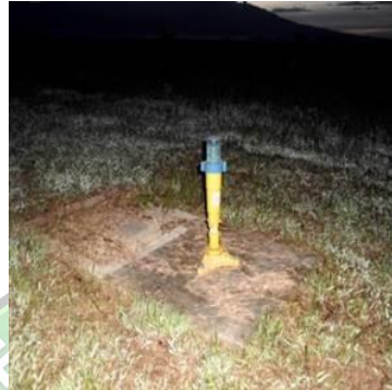
Gambar 3.1.5 6 Taxiway Edge Light
