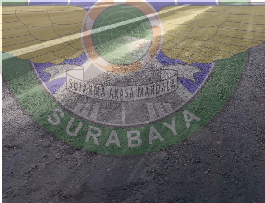
C.4 Lendutan dijalur roda ( Rutting )
