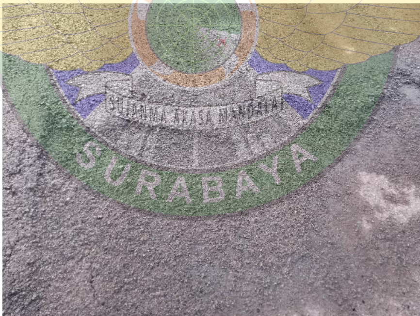
C.2 Pelapukan dan Butiran Lepas ( Weathering and Raveling )
