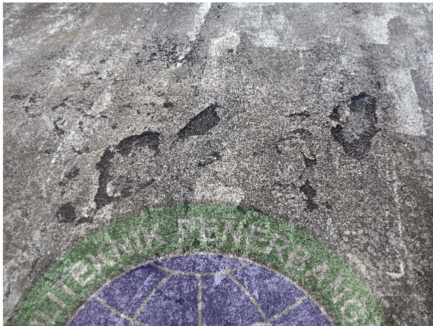
C.3 Lubang ( Pothole )
