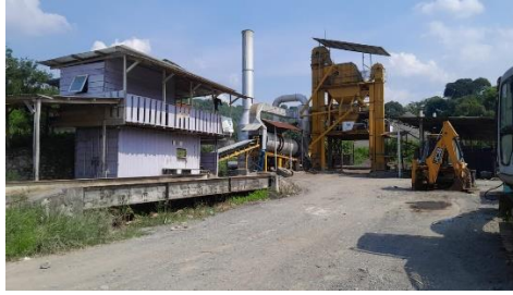
Gambar 4.26 Asphalt Mixing Plant (Sumber : Dokumentasi Penulis, 2025)
