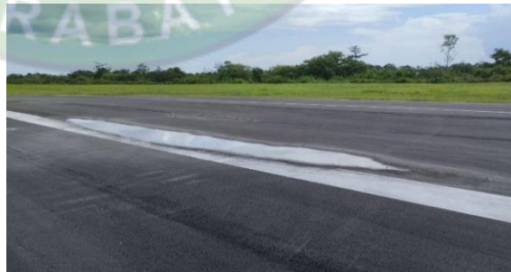
Gambar 4. 16 Water Ponding di area Runway 22 (Sumber: Penulis)
