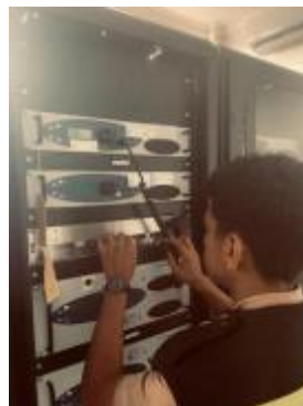
Gambar 4.3 Radio Main 118.1 Di ruang Tx
