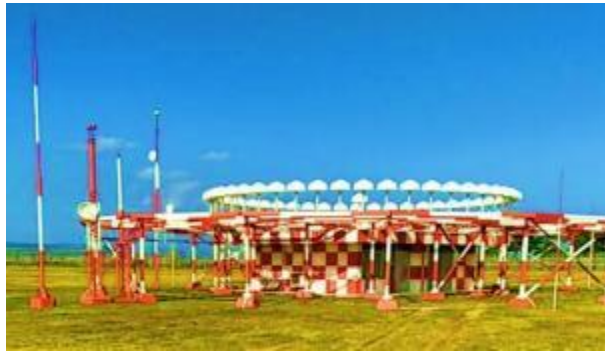
Gambar 3.19 Ground Station DVOR
