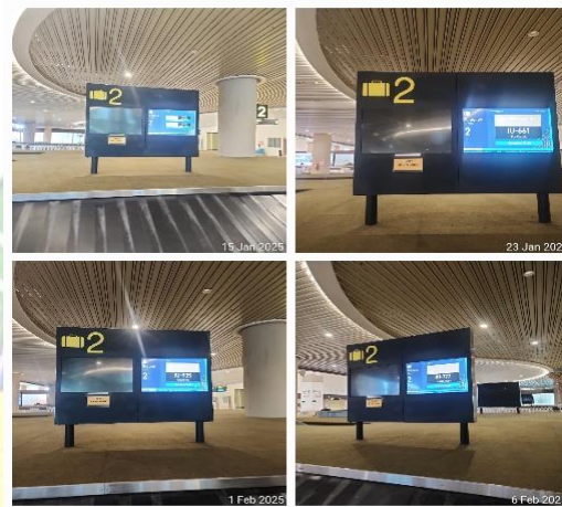
Gambar 4. 6 Display CCTV Pada Conveyor Belt di Area Baggage Claim Domestic
