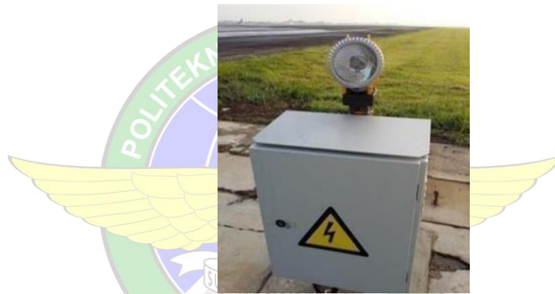
Gambar 2. 14 RTIL ( Runway Threshold Identification Lights ) Sumber: Dokumentasi penulis
