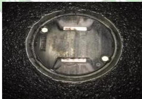
Gambar 2 8 Runway Centerline Light
