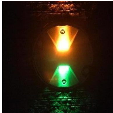
Gambar 2 11 Taxiway Centerline Light
