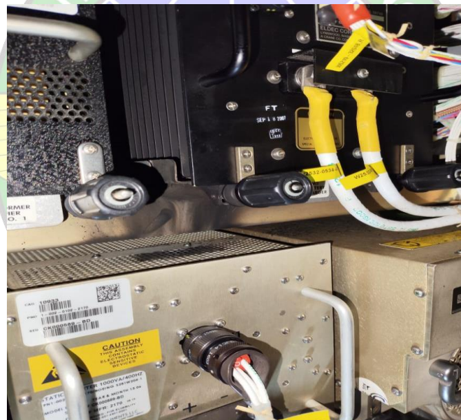
Gambar 4. 4 Burning Static Inverter
