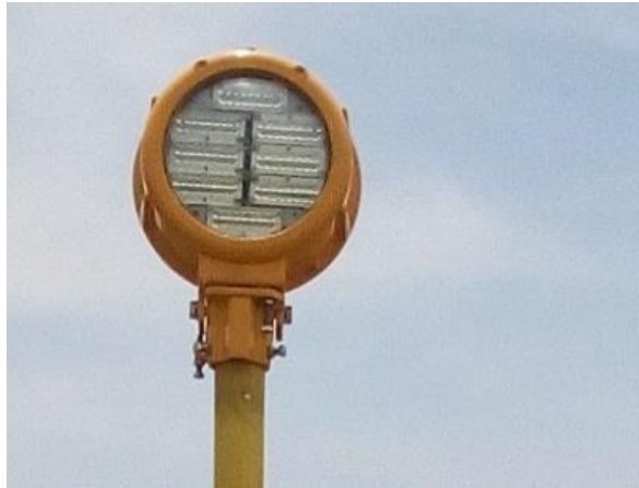
Gambar 2. 21 Runway Threshold Identification Light (RTIL)
