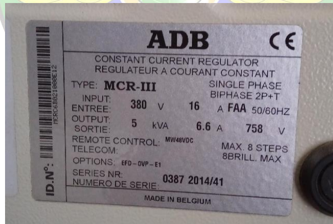
Gambar 2. 36 CCR Taxiway Edge Light Rangkaian C
