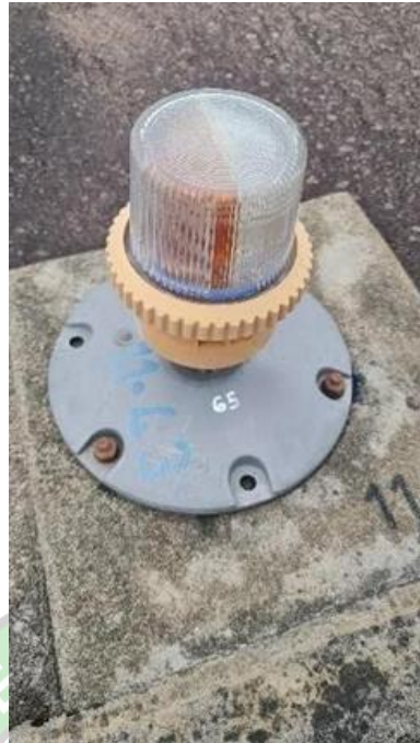
Gambar 2. 13 Runway Edge Light Elevated
