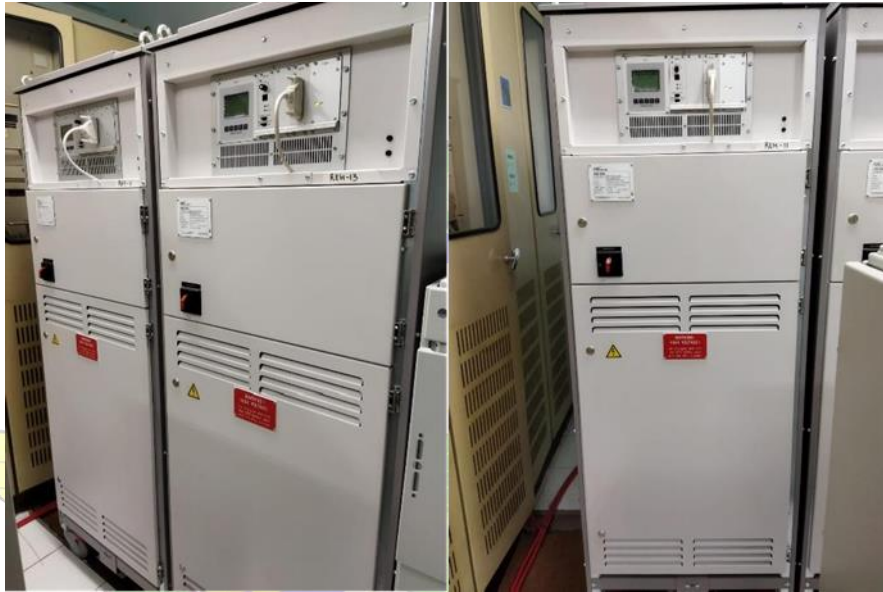
Gambar 2. 5 CCR Runway Edge Light & Runway End Light
