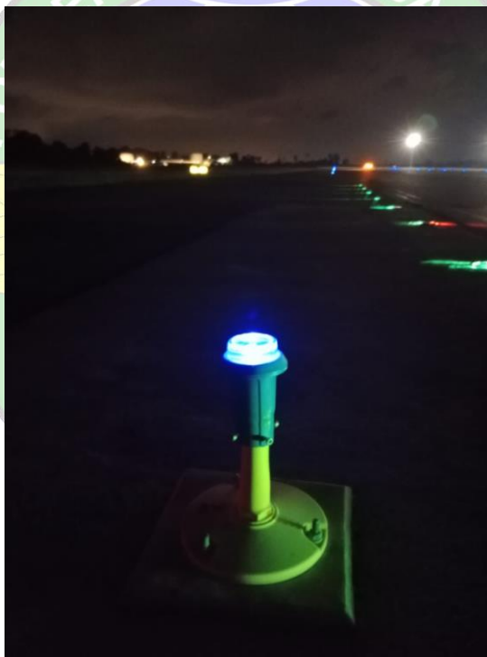
Gambar 2. 11 Taxiway Edge Light
