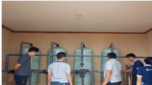
Gambar 4. 43 Mengontrol Masing-Masing Filter
