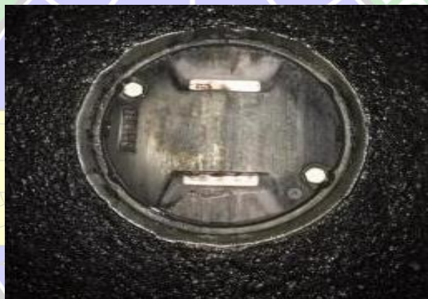
Gambar 2. 8 Runway Centerline Light
