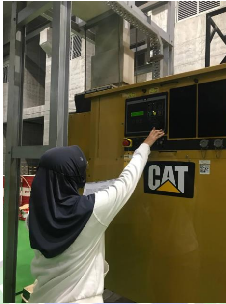
Pengecekan dan Run-up Genset
