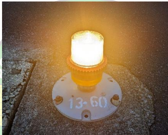
Gambar 3.1 Runway Edge Light Sumber : PT. Bandara Internasional Batam
