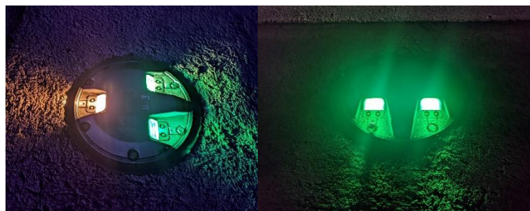
Gambar 2.17 Lampu Threshold Sumber: PT Bandara Internasional Batam
