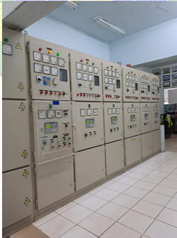
Gambar 2.10 Panel Automatic Change Over Switch
