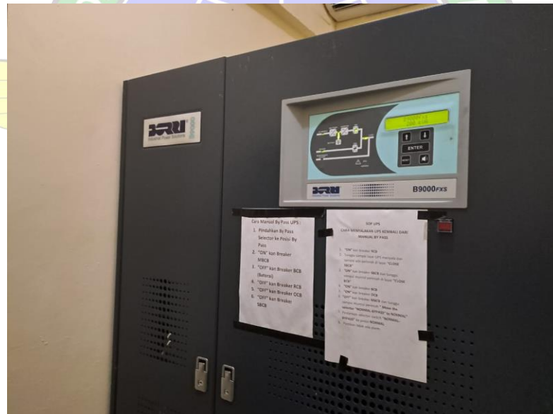
Gambar 2.11 UPS Power House Sumber: PT Bandara Internasional Batam
