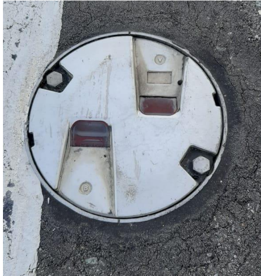
Gambar 2. 28 Runway Centreline Light
