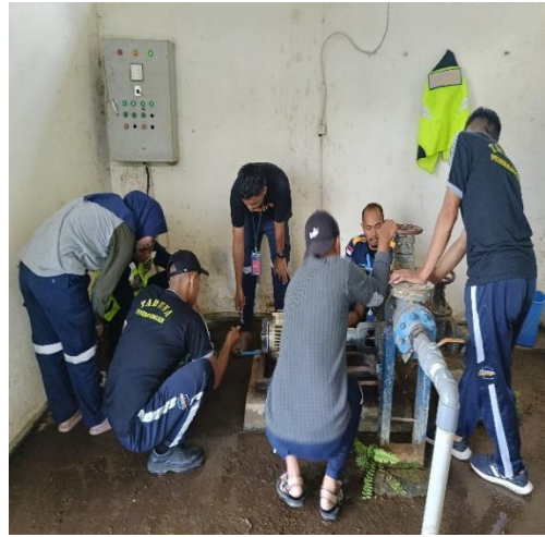
Maintenance Motor Sentrifugal
