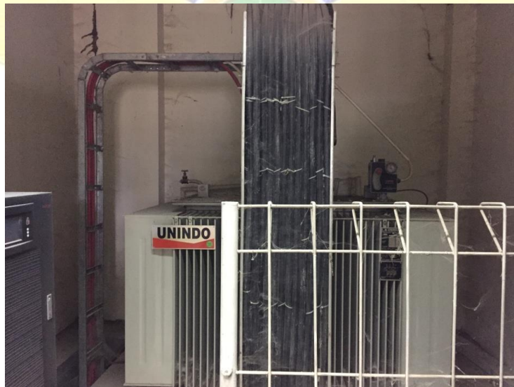
Gambar 4. 7 Transformator Step Down 2
