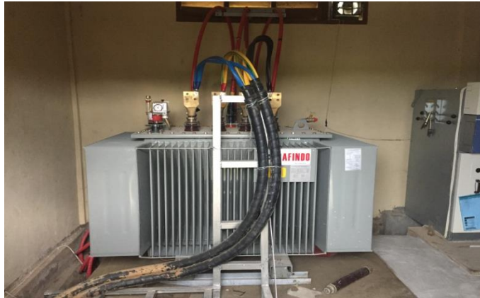
Gambar 4. 5 Transformator Step Up
