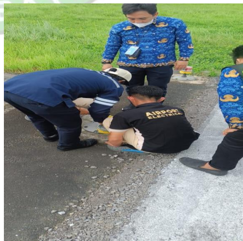
Maintenance Lampu Threshold
