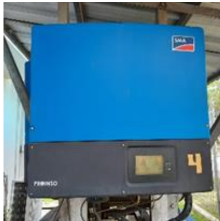
Gambar 3. 4 Inverter Solar cell
