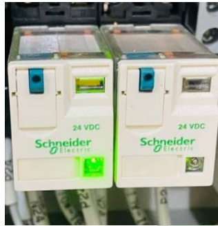
Gambar 3. 9 Relay 24 VDC Sumber: Bandara Supadio
