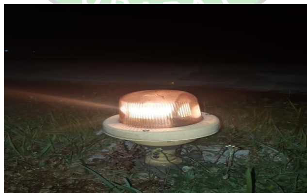
Gambar 2. 7 Runway Edge Light Elevated
