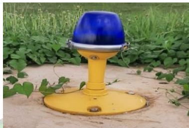
Gambar 2. 14 Taxiway Edge Light
