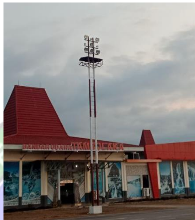
Gambar 2. 18 Apron Flood Light
