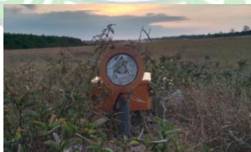
Gambar 2. 16 Runway Threshold Identification Light (RTIL)
