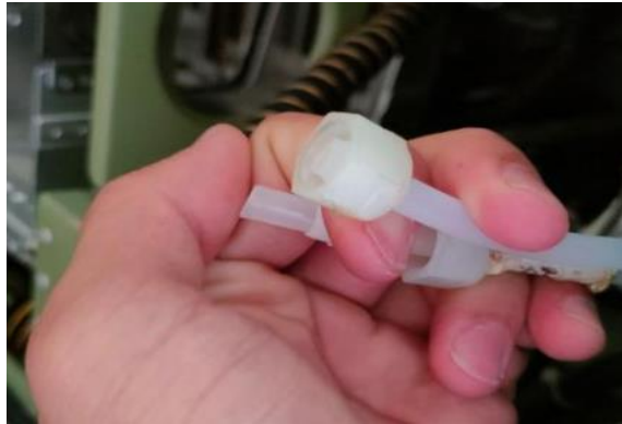
Gambar 4. 5 Leak On Pitot Line to GDC
