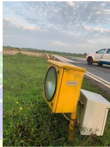
Gambar 2.4 Runway Threshold Identification Light
