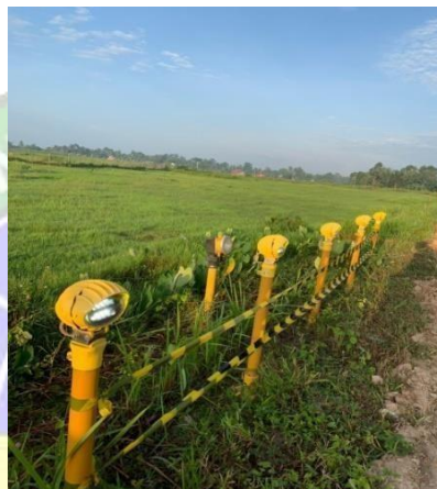
Gambar 2.2 Lampu Approach Light
