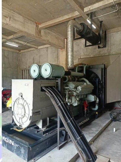
Gambar 2. 19 Genset 100 KVA (Leroy Somer)
