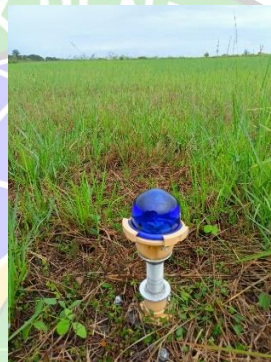
Gambar 2. 5 Taxiway Edge Light
