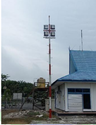
Gambar 2. 26 apron flood light
