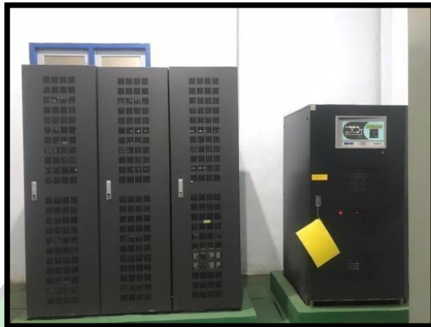
Gambar 2. 12 uninteruptible power supply 160 kVA
