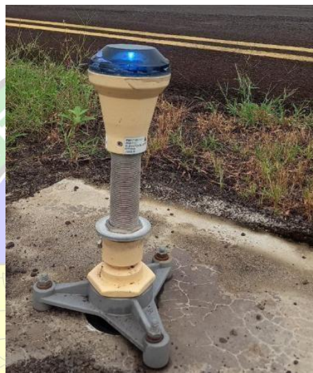
Gambar 2. 22 taxiway edge light
