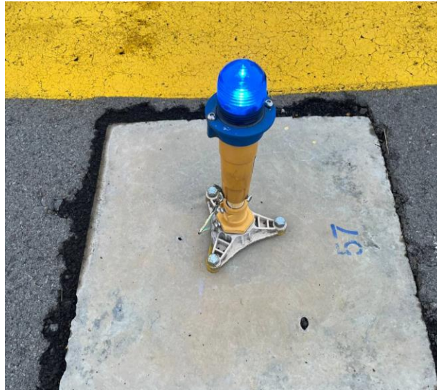
Gambar 2. 16 Taxiway Edge Light
