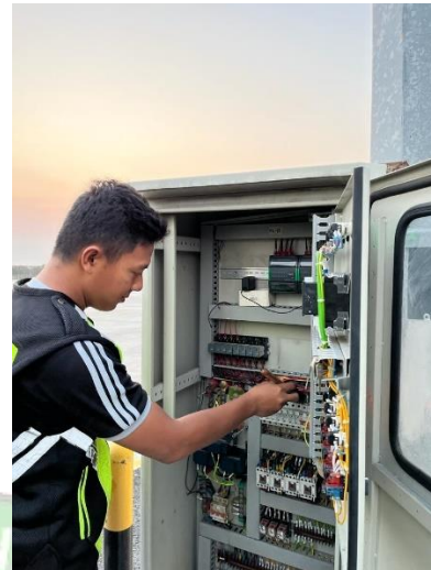
Perawatan Panel Floodlight
