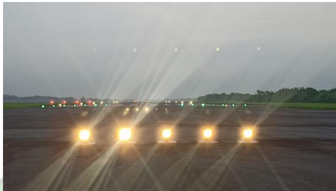
Gambar 2. 11 MALS ( Medium Aproach Lighting System )
