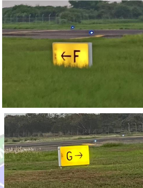
Gambar 2. 22 Taxiway Guidance Sign
