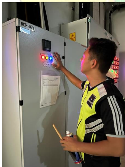
Perawatan Panel MDP 2A
