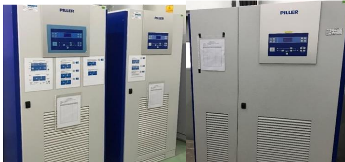
Gambar 2. 39 Uninterruptible Power Supply 100 KVA & 160 KVA
