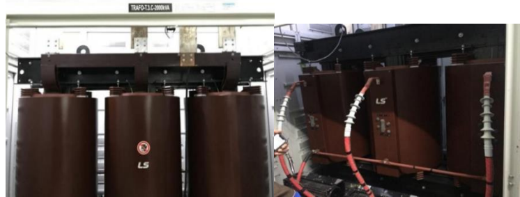
Gambar 2. 40 Transformator Step Down
