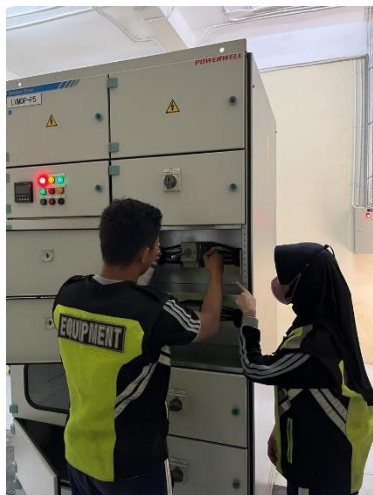
Perawatan Panel Pompa 5
