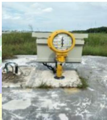
Gambar 4. 7 RUNWAY THRESHOLD IDENTIFICATION LIGHT (RTIL)
