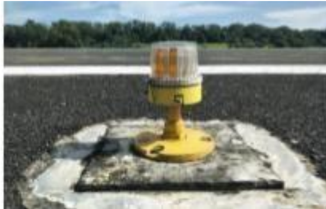
Gambar 4. 9 RUNWAY EDGE LIGHT ELEVATED
