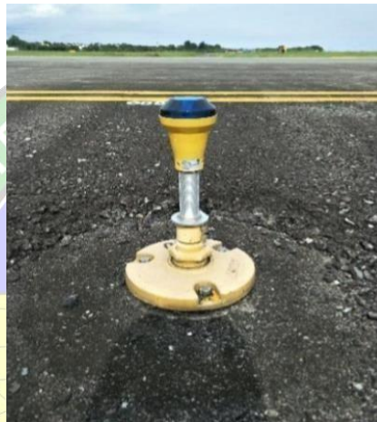
Gambar 4. 19 TAXIWAY EDGE LIGHT ELEVATED
