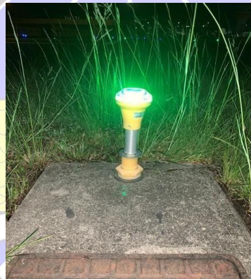
Gambar 4. 13 HELIPORT PERIMETER LIGHT
