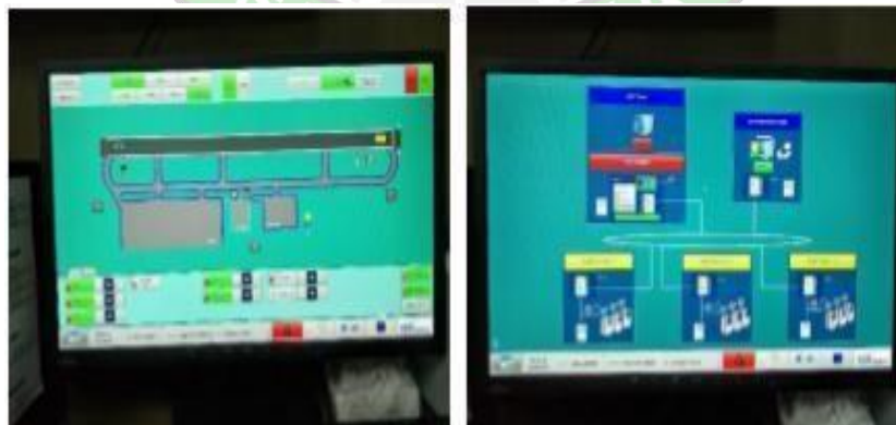
Gambar 4. 1 DISPLAY AIRFIELD LIGHTING CONTROL MANAGEMENT SYSTEMS
