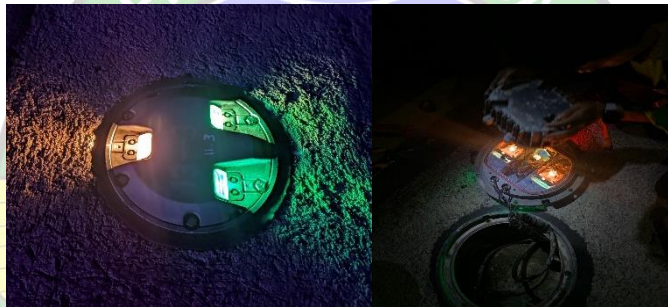
Gambar 2. 6 Lampu Threshold Sumber: PT Bandara Internasional Batam
