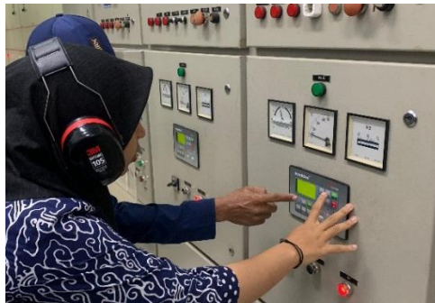
Gambar 2. 18 Panel Automatic Change Over Switch
