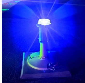
Gambar 2. 4 Lampu Taxiway Sumber: Data Peralatan BIB
