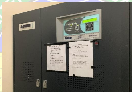
Gambar 2. 19 UPS Power House
