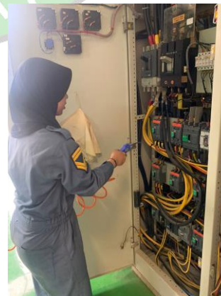
Perawatan Rutin Panel dan Sub panel di Terminal
