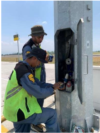
Perawatan Flood Light
