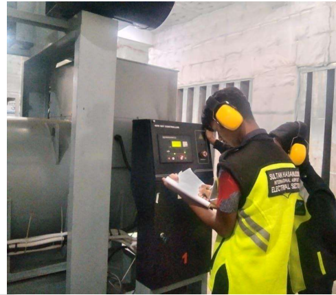
Monitoring Genset 2000 kVA Simulasi Black Out PLN
