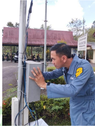
Pengecekan Panel Lampu PDU
