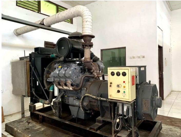
Gambar 2. 31 Generator Set 500 kVA
