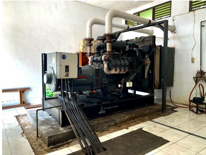
Gambar 2. 30 Generator Set 500 kVA
