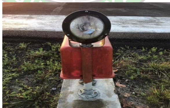
Gambar 2. 19 Runway Threshold Identification Light
