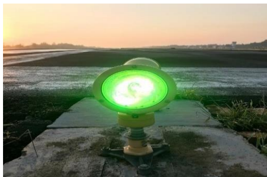
Gambar 2. 9 Lampu Threshold Elevated
