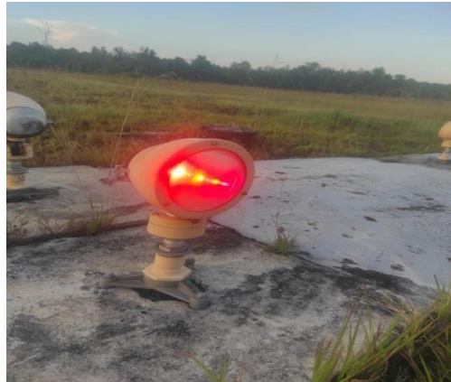
Gambar 2. 12 Runway End Light Elevated
