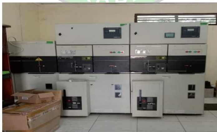
Gambar 2. 26 Panel Cubicle TM
