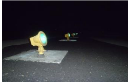
Gambar 2. 11 Wingbar Threshold Light Sumber: Bandara Internasional Husein Sastranegara
