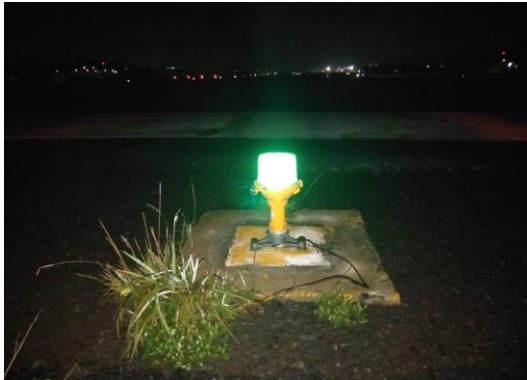
Gambar 2. 6 Threshold Light Elevated
