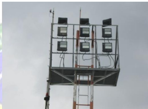
Gambar 2. 22 Apron Flood Light
