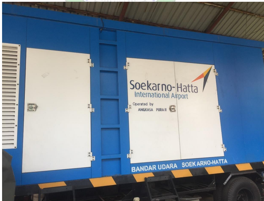
Gambar 2. 34 Mobile Genset 1000 kVA
