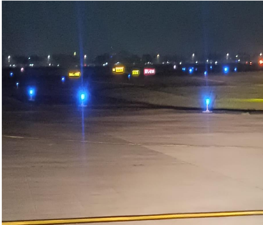
Gambar 3. 2 Taxiway Edge Light
