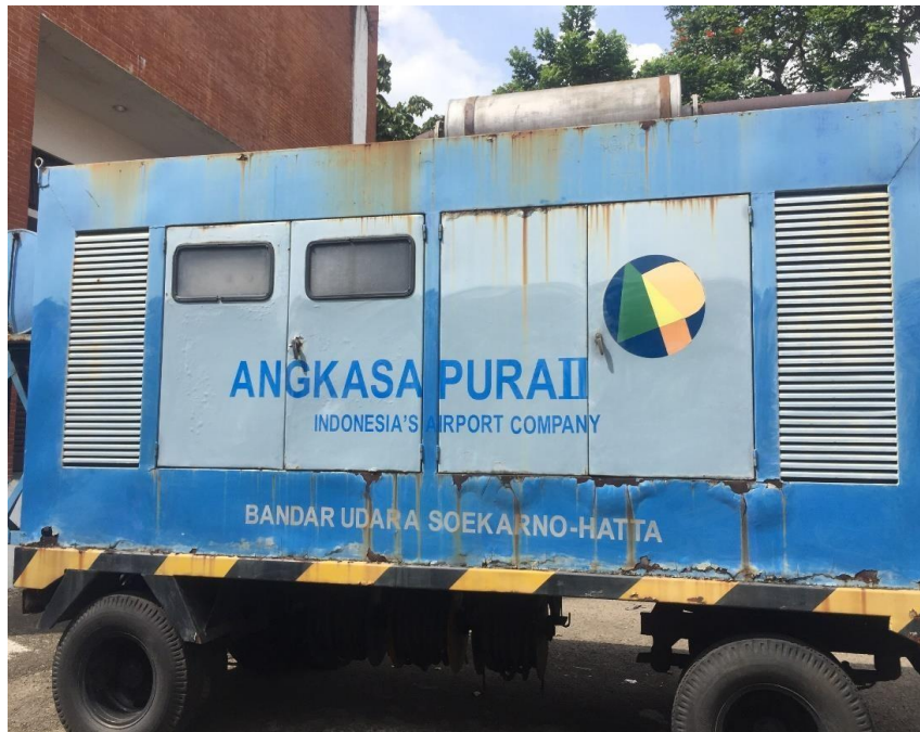
Gambar 2. 33 Mobile Genset 430 kVA
