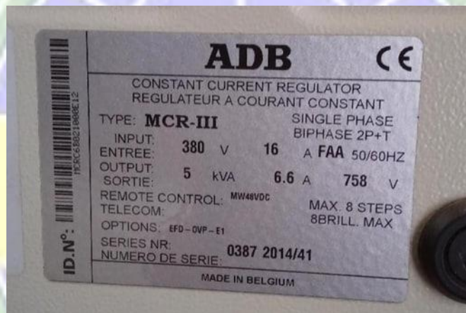
Gambar 2.36 CCR Taxiway Edge Light Rangkaian C
