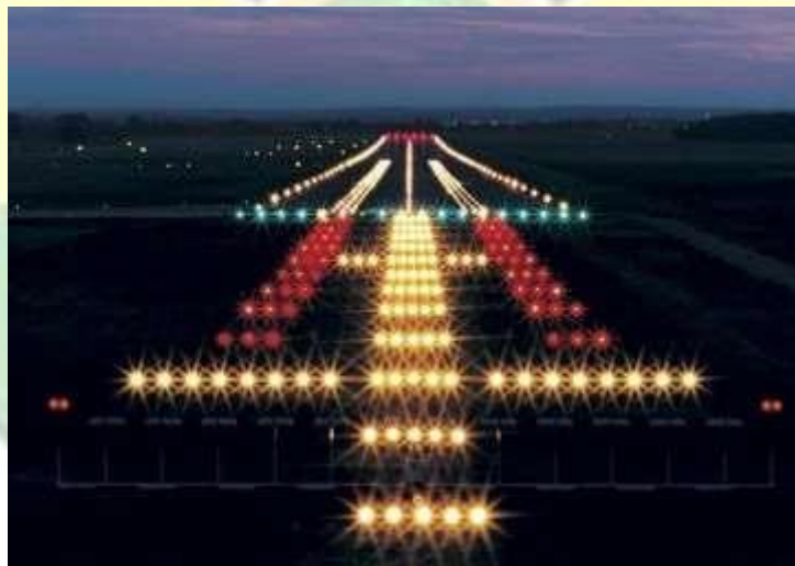
Gambar 3.1 Gambar Airfield Lighting System
