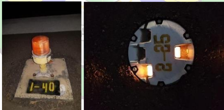
Gambar 2. 7 Runway Edge Lights
