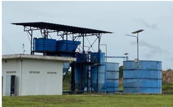
Gambar 4. 15. Ground Water Tank (GWT) (Sumber : Dokumentasi Penulis, 2024)
