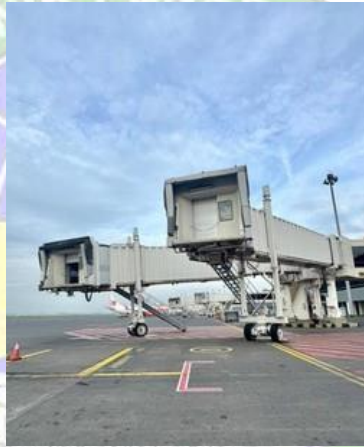
Gambar 3.5 Aviobridge (garbarata) dual tunnel
