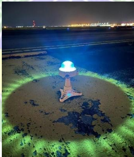
Gambar 2. 13 Taxiway Edge Light
