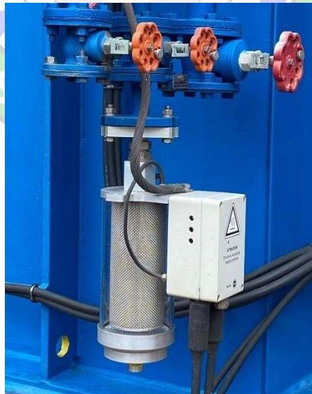
Gambar 3.17 Dehydrating Brether Trafo
