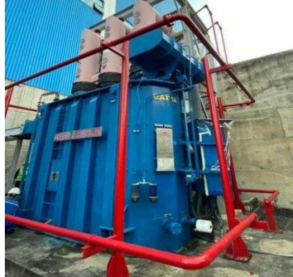
Gambar 3.9 Unit Auxiliary Transformer
