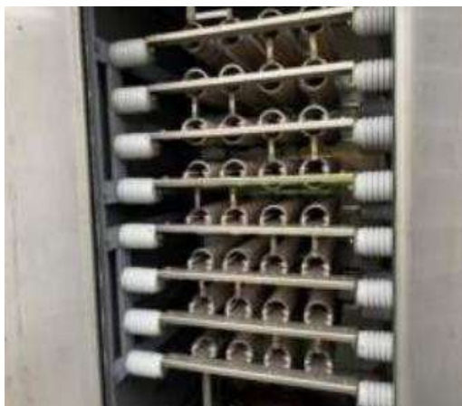
Gambar 3.16 Neutral grounding resistor trafo
