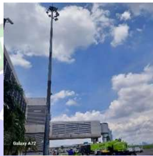
Gambar 2.10 Flood light T2 A3
