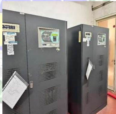
Gambar 2. 23 UPS Gardu R28
