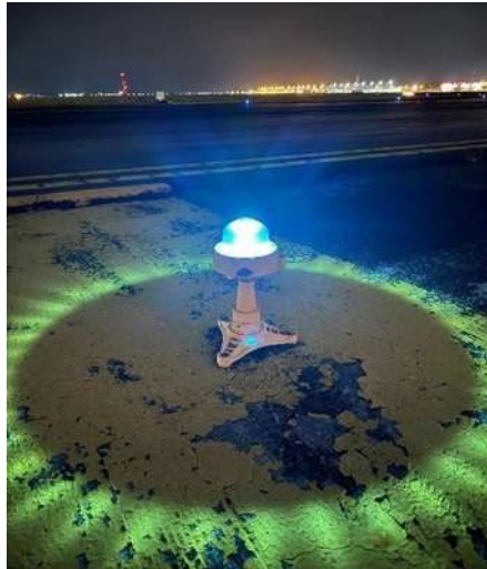
Gambar 2. 16 Taxiway Edge Light
