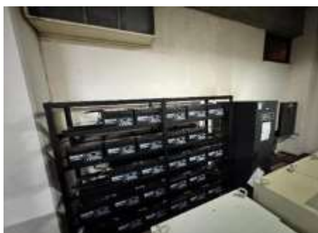
Gambar 2. 24 UPS Gardu R10
